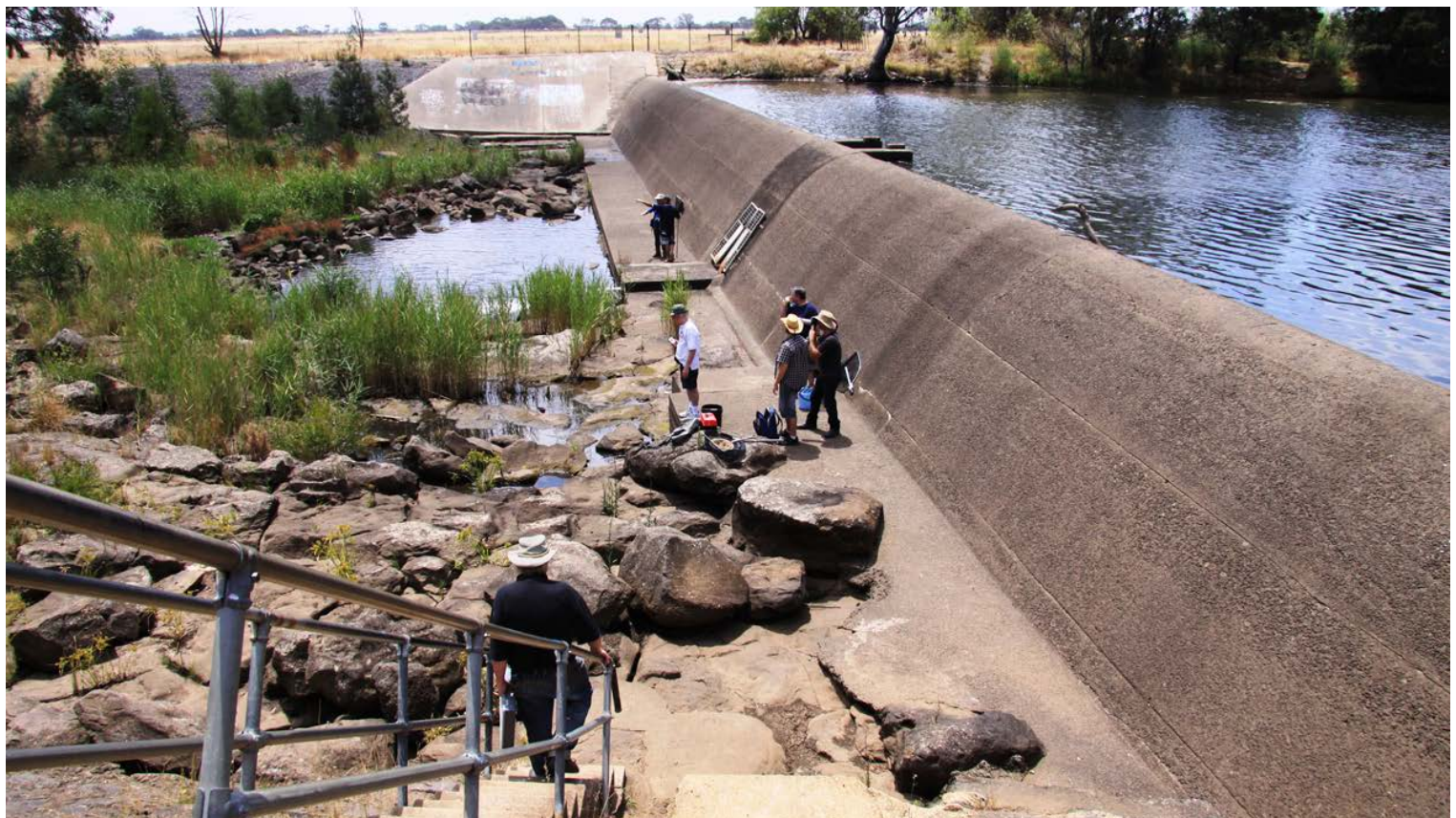
The weir at Centennial Park on the Werribee River. The weir is a major barrier to fishes movements/migration and several species congregate at the base of the wall. This photo was taken on an ANGFA Vic field trip in January 2014, and it will be great to go back after 9 years. Photo: John Lenagan
