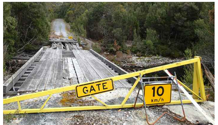
Sumac Road ends here, at this impassable bridge on Horton River. Travelling further south on this road is impossible, which is probably a good thing for the forest south of Horton River
